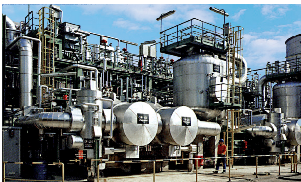
Figure 2. Processing capacity for sulfur recovery units (SRUs) may be increased through the addition of oxygen.
