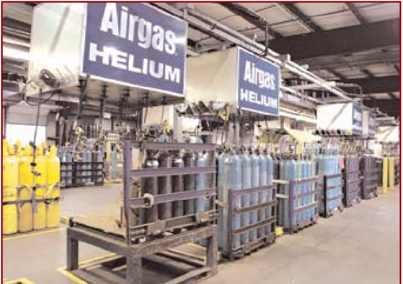
Airgas has 195 cylinder filling plants nationwide. Many, like this one in Cheshire, CT, are palletized fast-fill operations.
