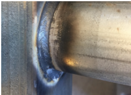
Good, sound weld
